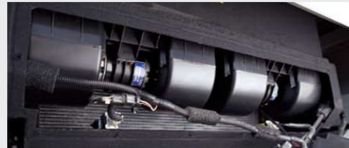
Sub heater under the floor
